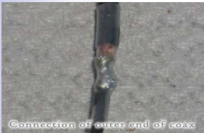
Photo C - Connection of outer end of coax section (further from center). Note that both center conductor and shield are connected to the wire.
