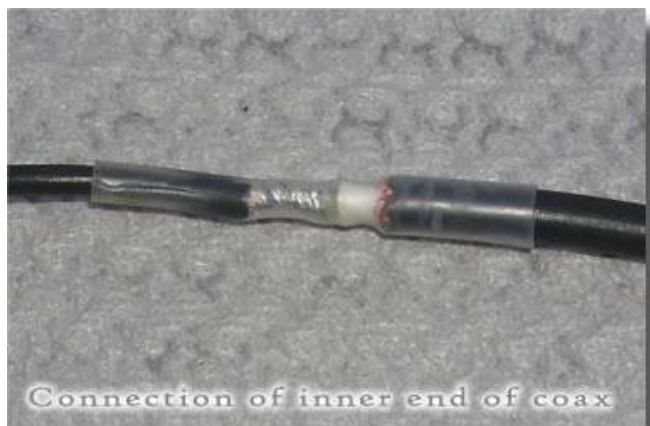
Photo B - Connection of inner end of coax section (closer to center). Note that only the center conductor is connected to the wire.
